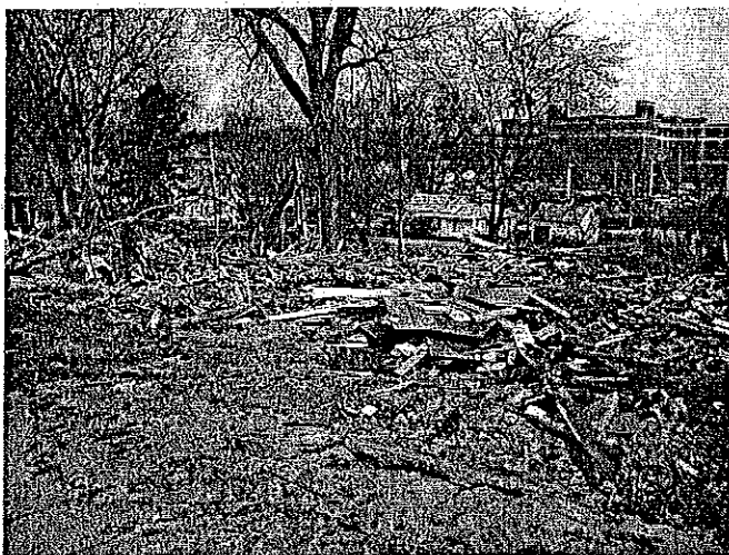
The landscape of the Gifford Park neighborhood has changed dramatically in the last few weeks with the demolition of nearly all the houses between 30th -32nd, California to Webster St. Creighton University is conducting the demolition as part of its campus expansion project.
